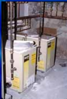
Weil-McLain GV4 Boilers
